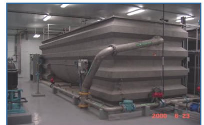
▲ Village of South River, ON Design Flow: 1680 m 3 per day
