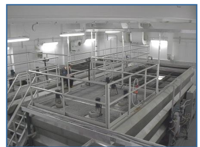
▲ Town of Port Carling, ON Design Flow: 1584 m 3 per day
