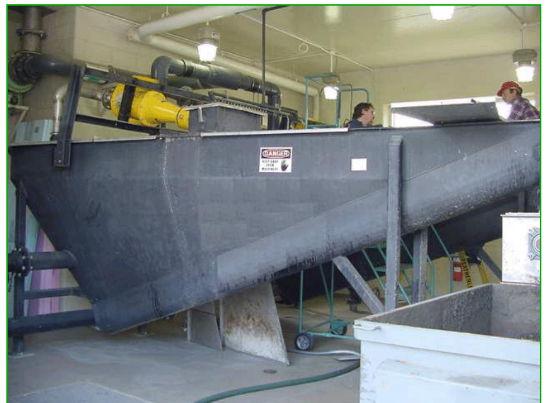
▼ Screw Grit Classifier c/w Hydro-cyclone Corbett Creek WWTP Ontario, Canada
