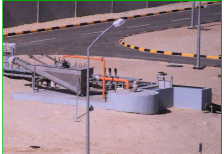
▲ Wafra WWTP Kuwait
