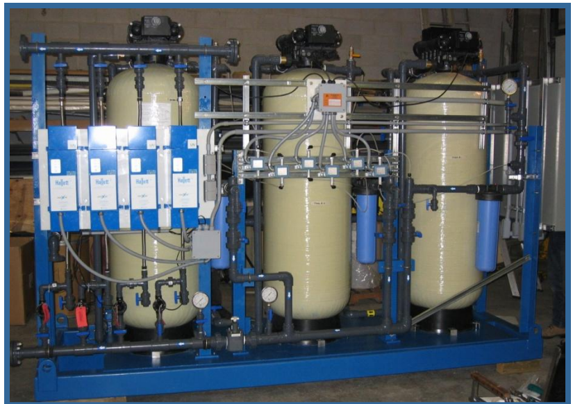
NR - Pressure Filtration Skid OPG Lennox Power Generation Station Bath, Ontario Design Flow Rate: 197 m 3 per day
