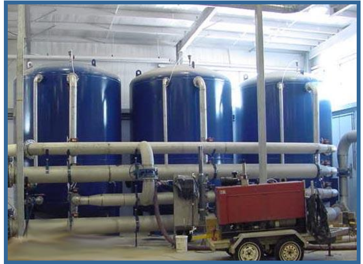
▲ NR - Pressure GAC Tower South Chatam, Ontario Design Flow of each tower: 7600 m 3 per day
