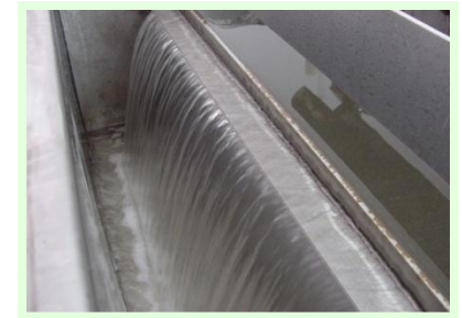
Effluent from DIFLOAT™ DAF System
