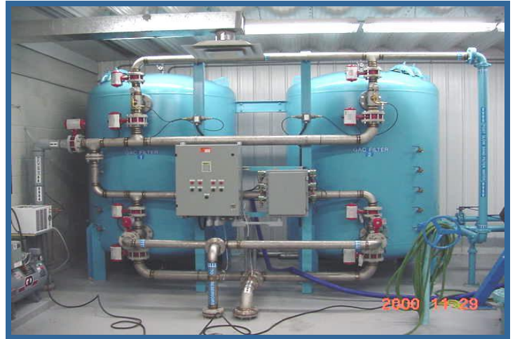
▲ NR-GAC Filter - North Caribou, First Nation, Ontario, Canada Design Flow 1080m 3 per day
