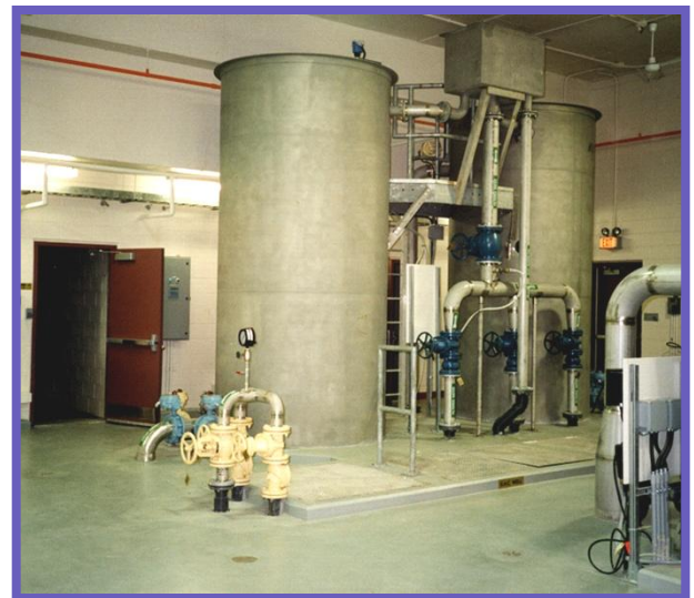
NR-GAC Tower , installed in 1999 at Echo Bay, Ontario, Canada, to remove organic contaminants
