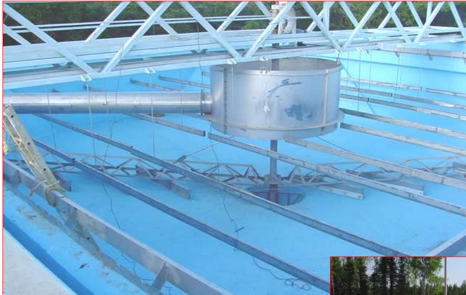
▲ NR- Conventional Clarifier – Belize City WTP Belize, Central America Design Flow: 14,000 – 20,000 m 3 per day
